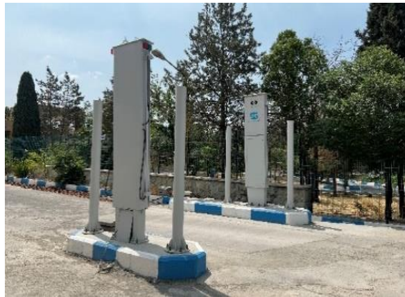
Fig. 1. Radiation portal monitor system
