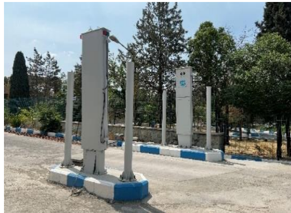
Fig. 1. Radiation portal monitor system
